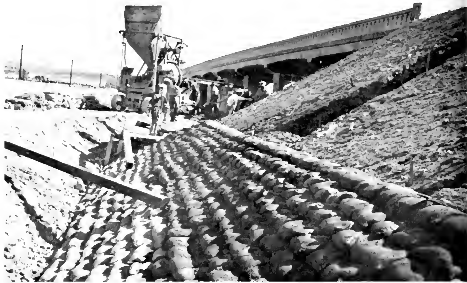
Sacked concrete riprap was placed at the ends of the bridge over San Gorgonio Wash to protect the adjoining embankments from storm damage
